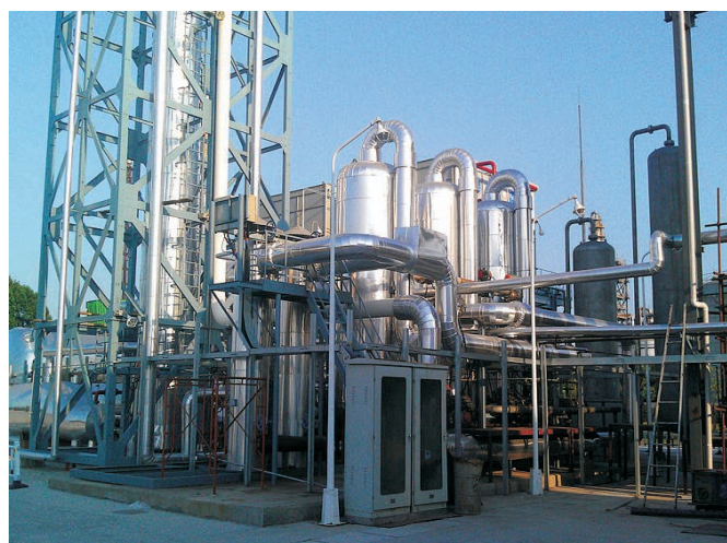
CO 2 Recoverd & Purified Plant (200,000 ton/y)
